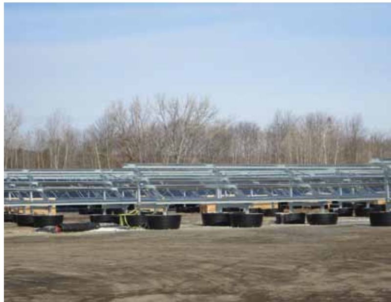
Photovoltaic panels at Truck Stop Solar project on Route 102 west of town. A "ballasted racking system" was used as an alternative to driving posts into contaminated soil at the brownfield site. Photo by John Parker.
