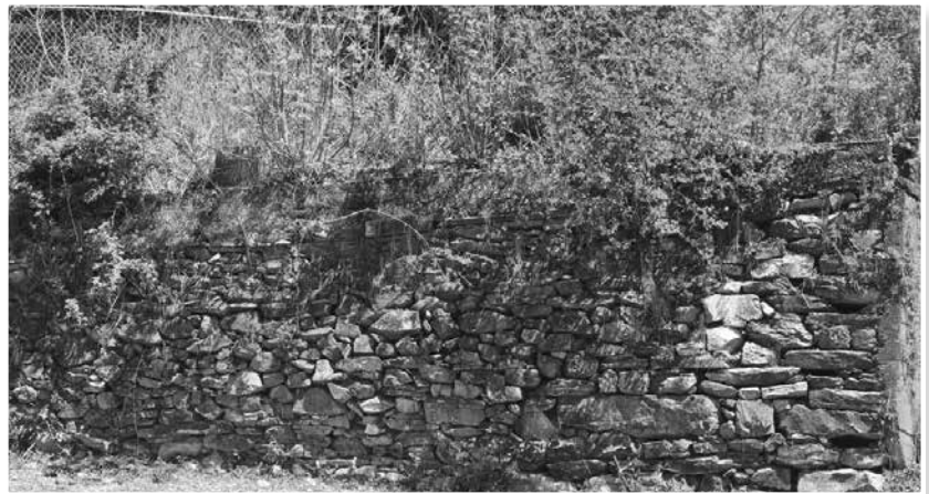
Foundation wall at rear of parking lot. Photo courtesy of Bob Salerno
