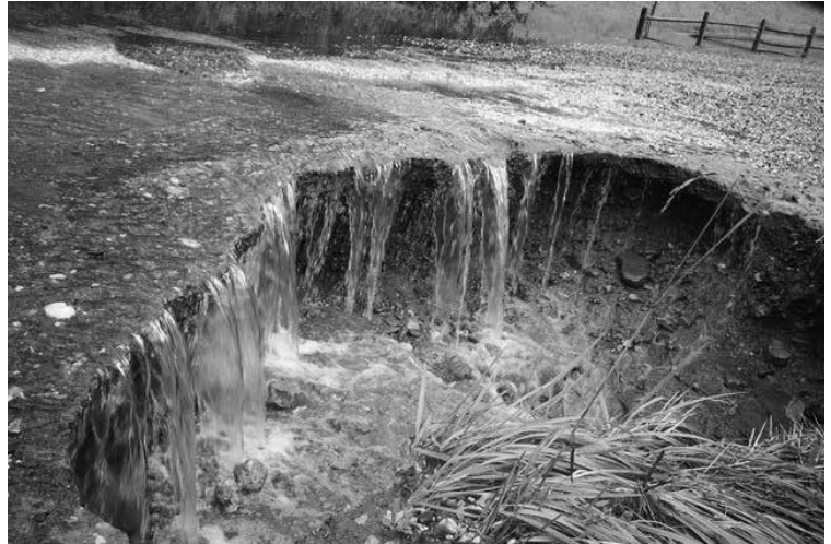
Washed out roadway on West Road
