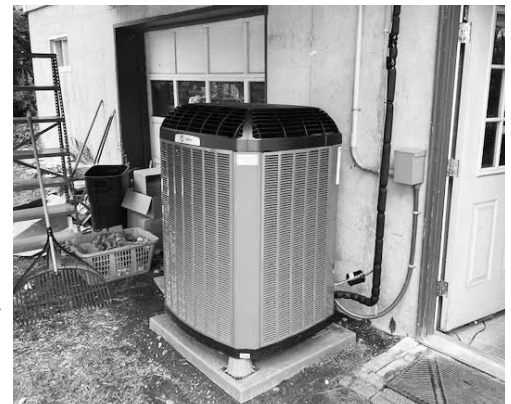
Our new heating source: an electric heat pump. Photos courtesy of Shaker Mill Books
