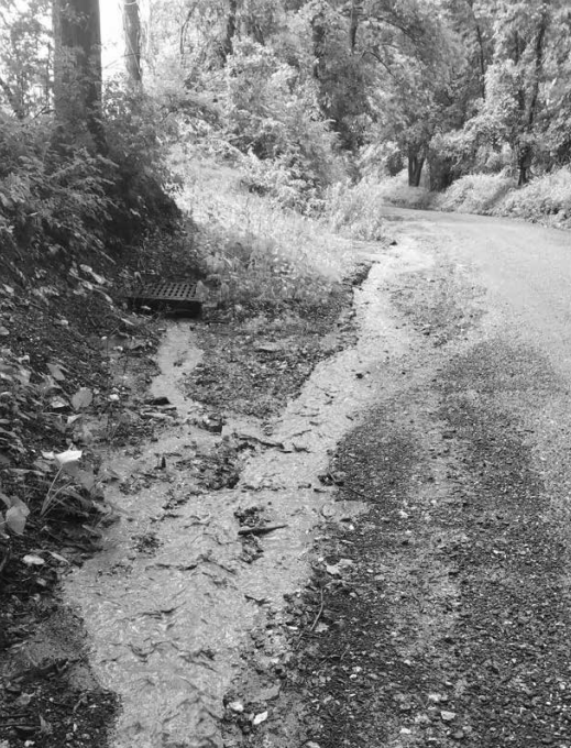
Runoff on Maple Hill Road. Photo courtesy of BRPC
